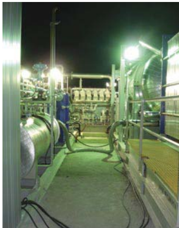
Mobile Evaporator treating Barnett fracture flowback water for recycling Source: Onsite Water Treatment , 2006.
